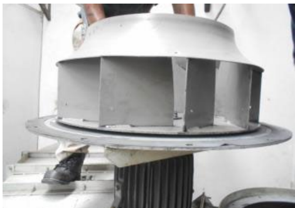
Fig. 5c. Impeller after cleaning
