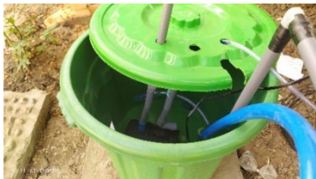
Fig. 3. The hydroponic nutrient reservoir is connected to PVC pipes to channel the nutrient solution to the topmost section and then back to the reservoir
