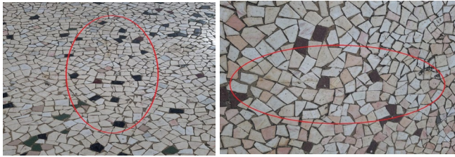
Fig. 1. Cracks noticed and wider from 0.50 mm to 3 mm on terrace roof
