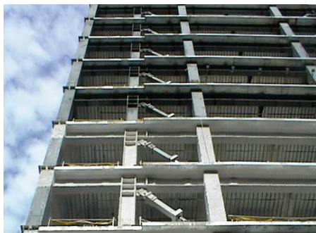
Fig. 3. Dampers in building
