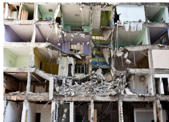
Fig. 5. Earthquake affected building
