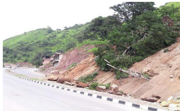
Fig. 2. Landslides in Joginder Nagar
